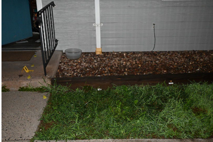
[Bullet defects in landscape timber]
