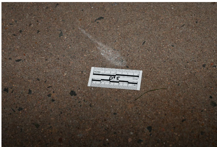
[Bullet defect in concrete front stoop]
