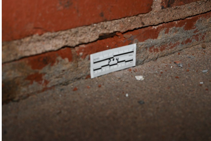
[Bullet defect in brick wall]
