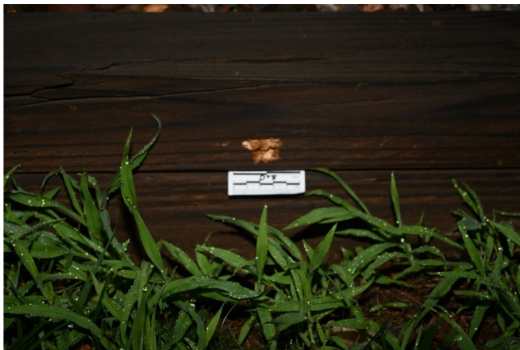
[Second bullet defect in landscape timber]
