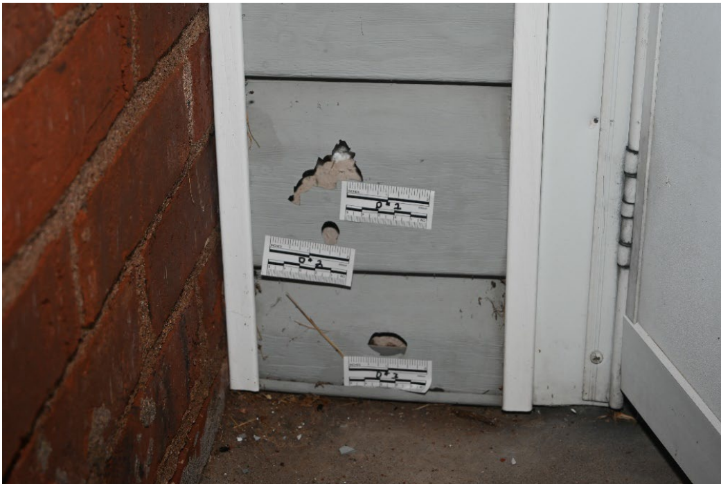
[Bullet defects in siding of apartment]
