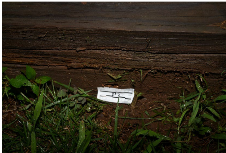
[Bullet defect in landscape timber]
